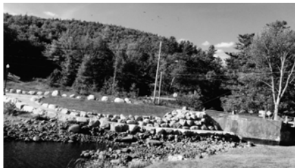
New Bridge and Dam constructed over the Summer - Bridge Opened in November
